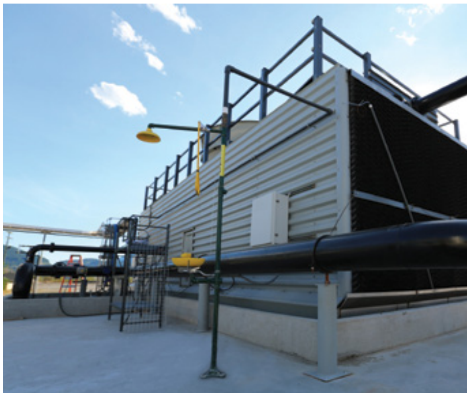
CE’s pilot scale air contactor in Squamish, B.C. This device can scrub roughly 1 tonne of CO 2 per day from the air. Carbon Engineering photo
